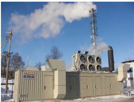
City boiler room Krasnopolje, Belorussia (2010)
